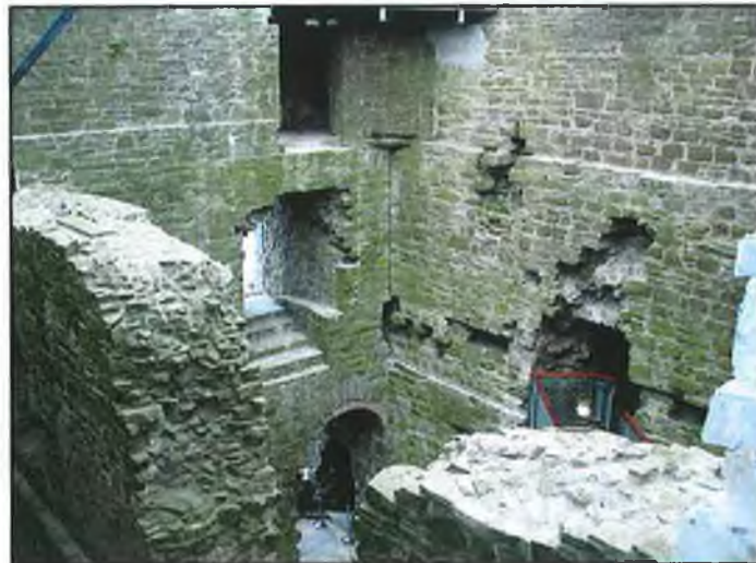
FIG. 6.17 Part of spine wall and features on hall (east) side of keep viewed from southwest.
