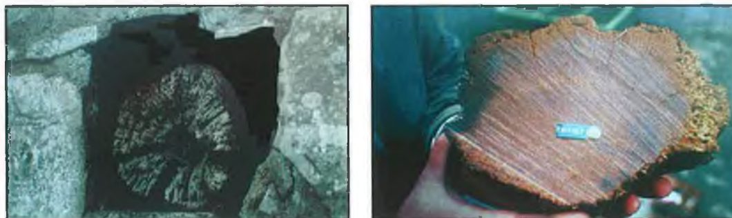
FIGS 6.42-3 Putlog hole and timber (in situ) in keep; sample of timber removed for dendrochronological analysis. Source: Condit, 'Rings of truth at Trim Castle', pp 30, 32.
